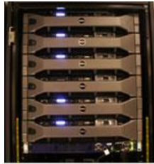
Dell™ PowerEdge™ R815 11-node cluster
